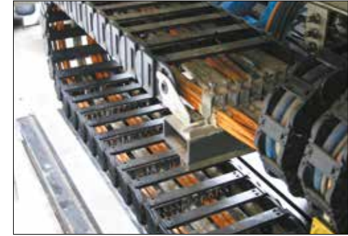
Top condition even after 9 years: e-chain® in a high-precision lathe and grinding machine.
